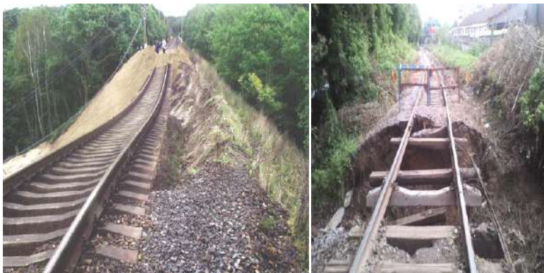
Fig. 1: The sudden destruction of the subgrade of the railway as a result of natural factors
