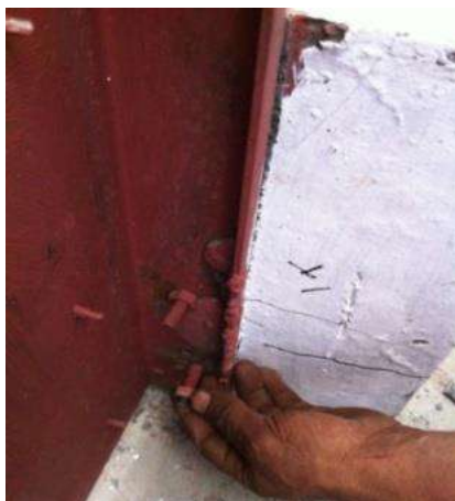
Fig. 6(a): Bending of the bolts.
