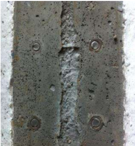
Fig. 6(c): Failure in concrete around the bolts.
