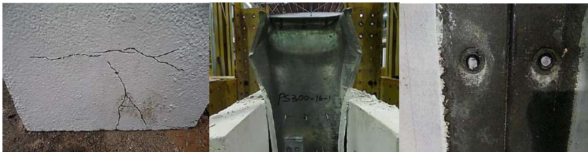
(a) Concrete Cracking and Crashing
