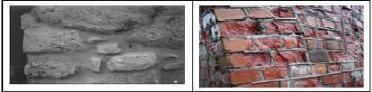
Fig. 2. Show the weakness of Components of the brick and mortars brick walls of the historical influence of long-term deterioration
